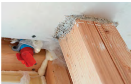
Aerosolized air-sealing. Many builders have turned to the AeroBarrier system to either bolster their already diligent air-sealing efforts, or as their primary strategy. The system uses a blower door to direct aerosolized water-based sealant to air leaks, where it accumulates and seals the gaps.
