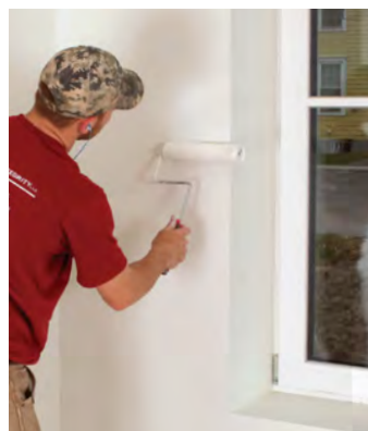
Semi-permeable materials (Class III vapor retarders) , including most cured latex paint, plywood, and OSB, have a perm rating greater than 1 and up to 10.
