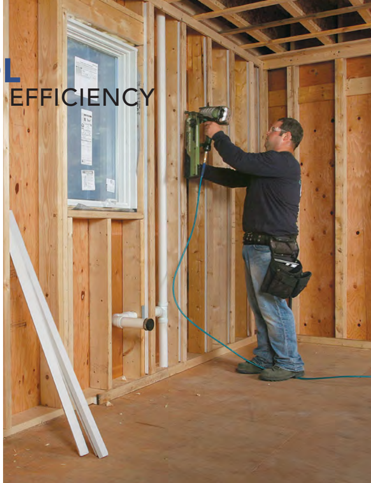
Keep ‘em separated. An effective temperature control layer includes a thermal break at the framing because wood is a poor insulator. An alternative to double-stud walls and continuous exterior insulation is to fur out the framing on the interior with strips of rigid-foam insulation.
