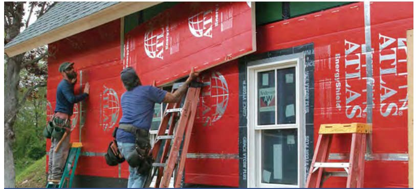
Vapor-impermeable materials (Class I vapor retarders) , including foil-faced insulation, polyethylene sheeting, and glass, have a perm rating of 0.1 or less.
